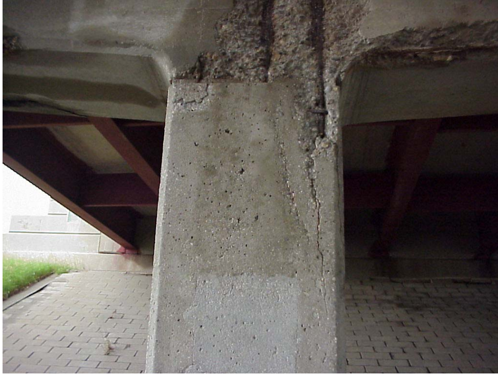
Figs. 5.1 Column condition before surface repairs
