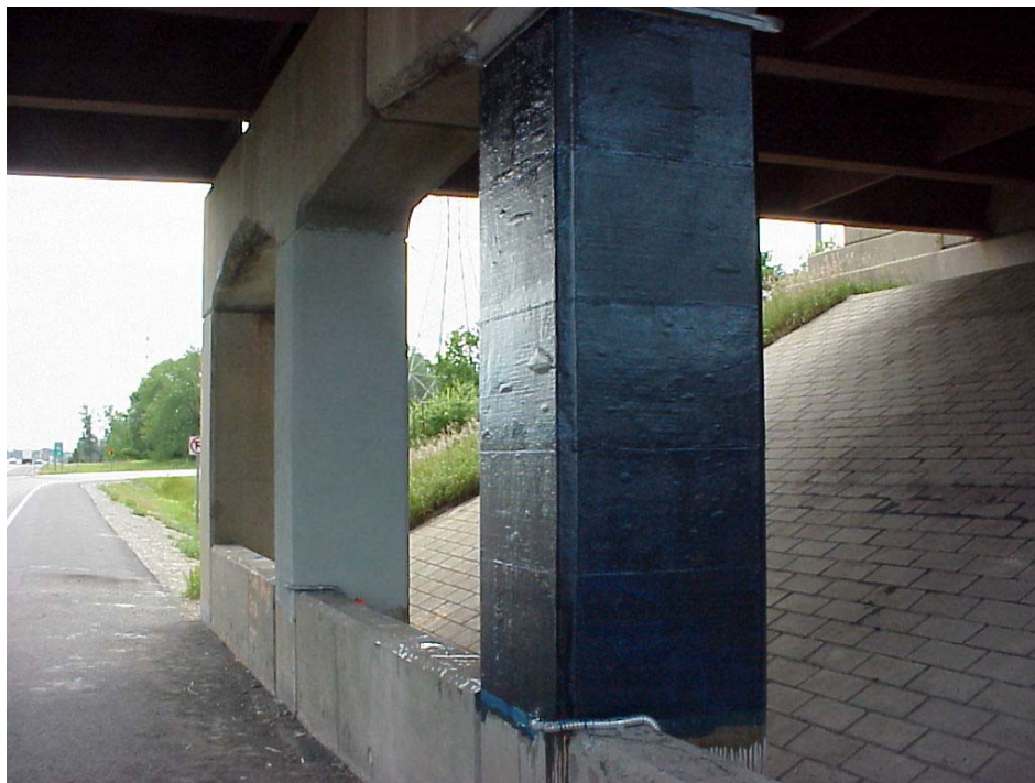
Fig. 5.6 Completed installation of glass and carbon wraps (glass wrapped column in the background with top coat and final paint layers applied).
