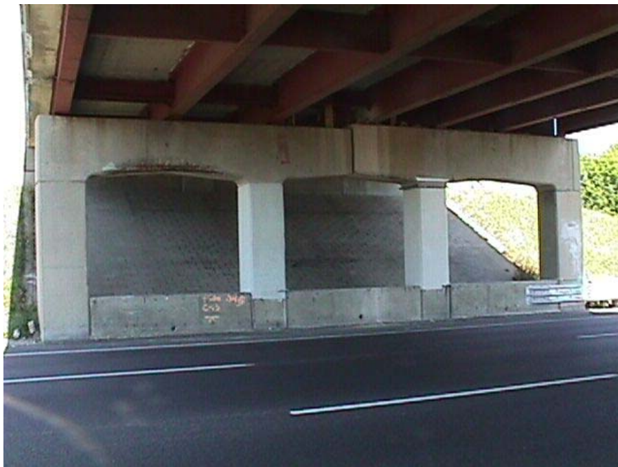
Fig. 5.8 Control (far right), carbon-wrapped (right) and glass-wrapped (left) columns under eastbound overpass (S10)
