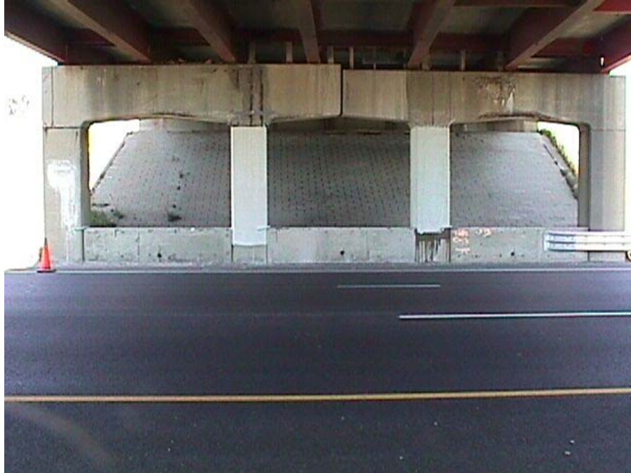
Fig. 5.7 Control (far left), carbon-wrapped (left) and glass-wrapped (right) columns under westbound overpass (S09)
