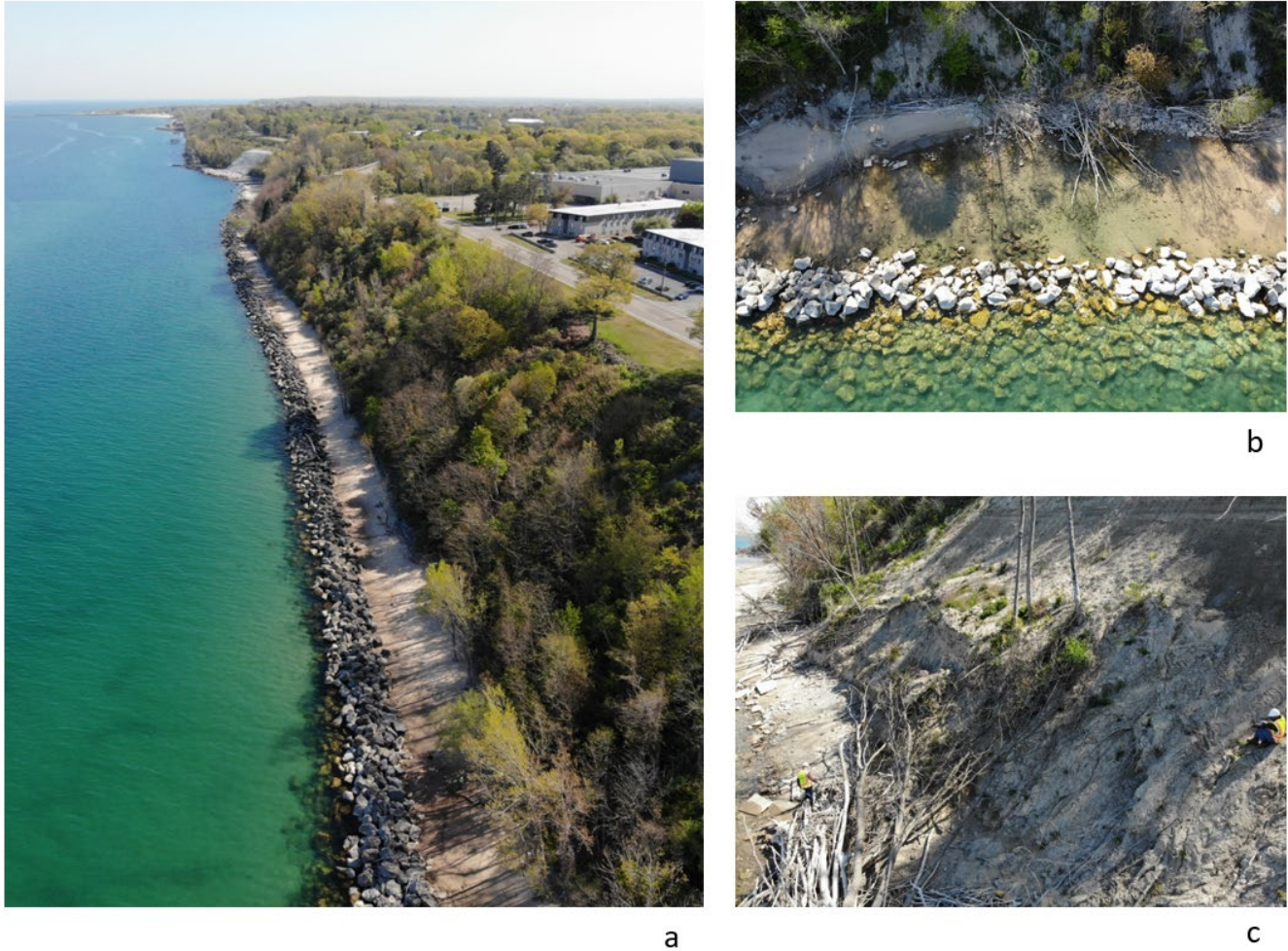
Figure 4-13. Drone imagery of I-94 BL St. Joseph, May 2021, showing a) the roadway in relation to the bluff and existing mitigation measures, b) existing state of rip-rap mitigation measures, and c) evidence of slope failure.
