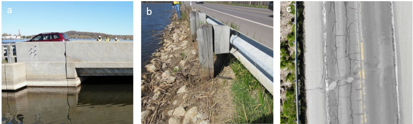
Figure 4-3. Damage as captured in May 2021. a) high water mark on bottom of bridge beams. b) debris from high water and rotting of guardrail posts, c) ruts and cracking on pavement.
