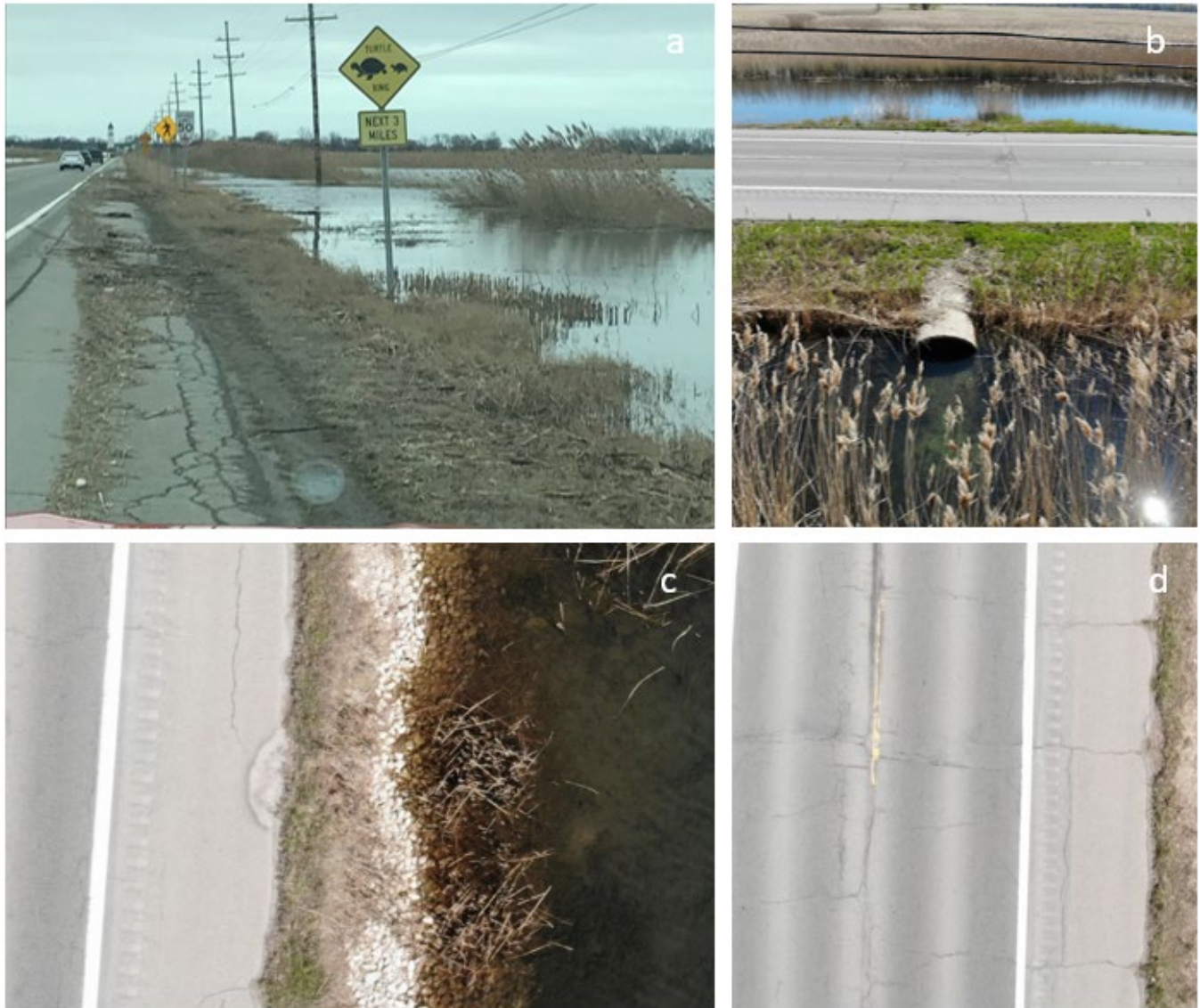
Figure 4-7. Historic flooding and current condition of roadway. a) debris showing extent of high water that has since receded (as well as an unapproved “turtle crossing” sign), b) a pipe culvert, one of the two culverts along the 5,800 feet considered, c) evidence of muskrat damage on the shoulder, d) typical cracking and rutting of this section of roadway.
