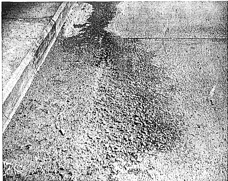
▲ FIGURE 15. VERY DEEP SCALING ON SPAN 11 ON OUTSIDE NORTHBOUND LANE.
