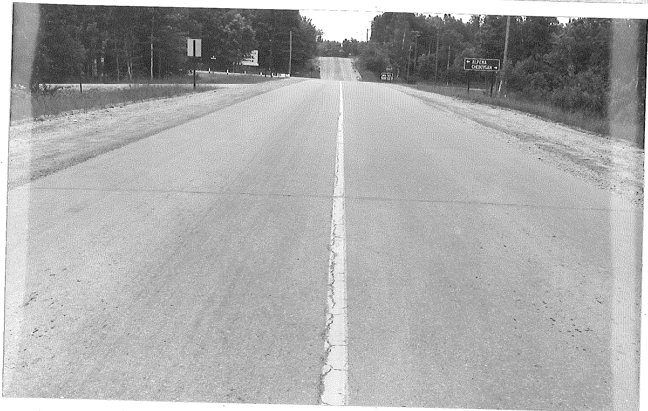
Figure 7. West end of resurfaced project, over section originally constructed as control, without HP-7. Note reflection cracking over longitudinal and transverse joints (bottom).
