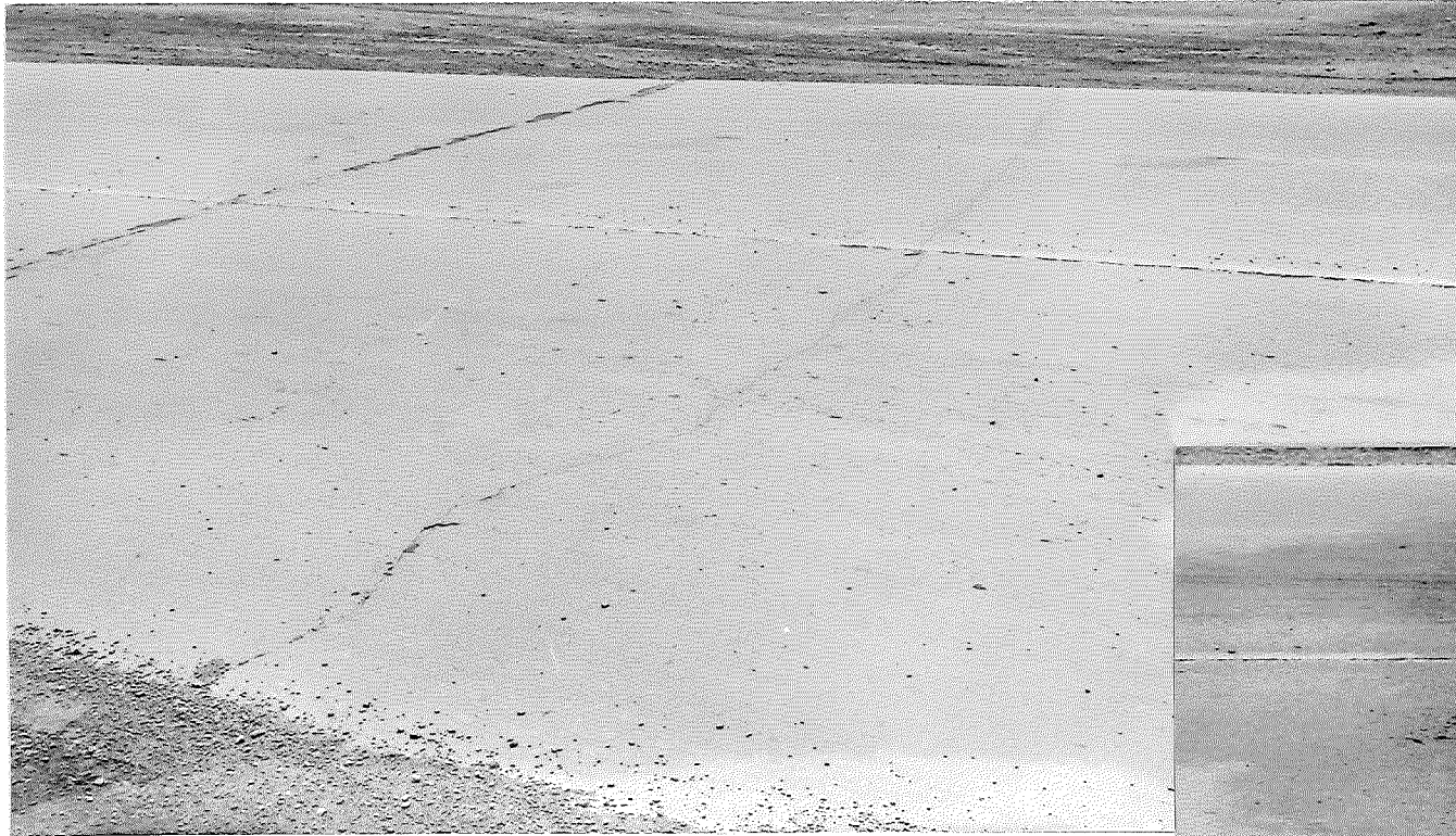
Figure 2. Typical transverse crack (above).
