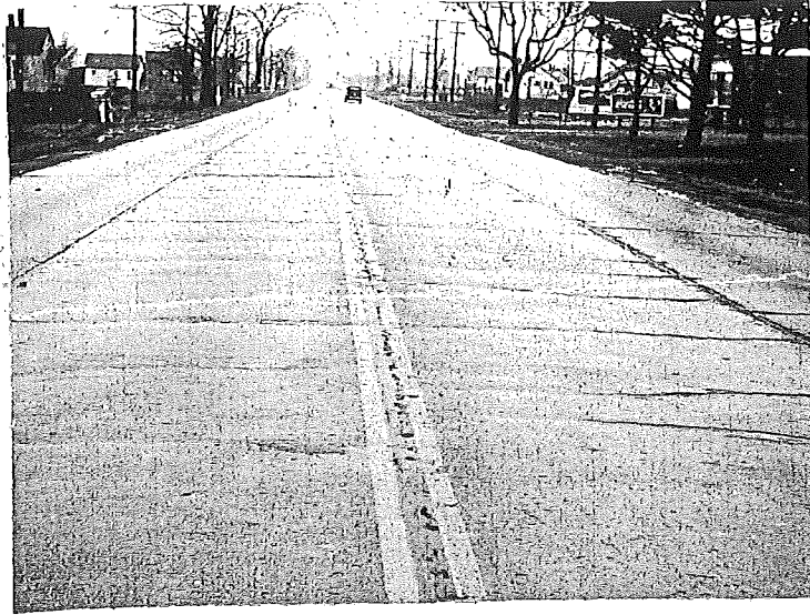
Figure 3. Project 25-5, Cl, 1-26-44. General view of pavement showing comparative transverse cracking of the recapped section in center to the widened section. Pavement 13 years old.
