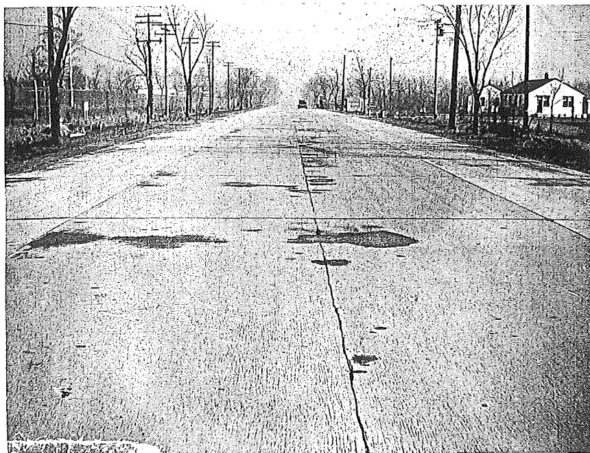
Figure 8. Project 50-30, C2, 1-26-44. General view showing recapped section in center and widening on sides. All surfaces were in excellent condition. View also shows contrast in color of surfaces. Concrete on recapped section was colored by using Emulsified Carbon Black. Pavement 2 years old.
