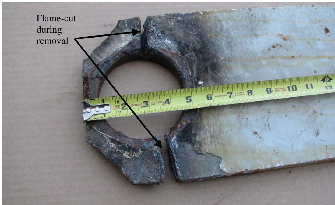
Figure 3 Salvaged link plate from R02-39022 with 38 percent section loss behind pin-hole
