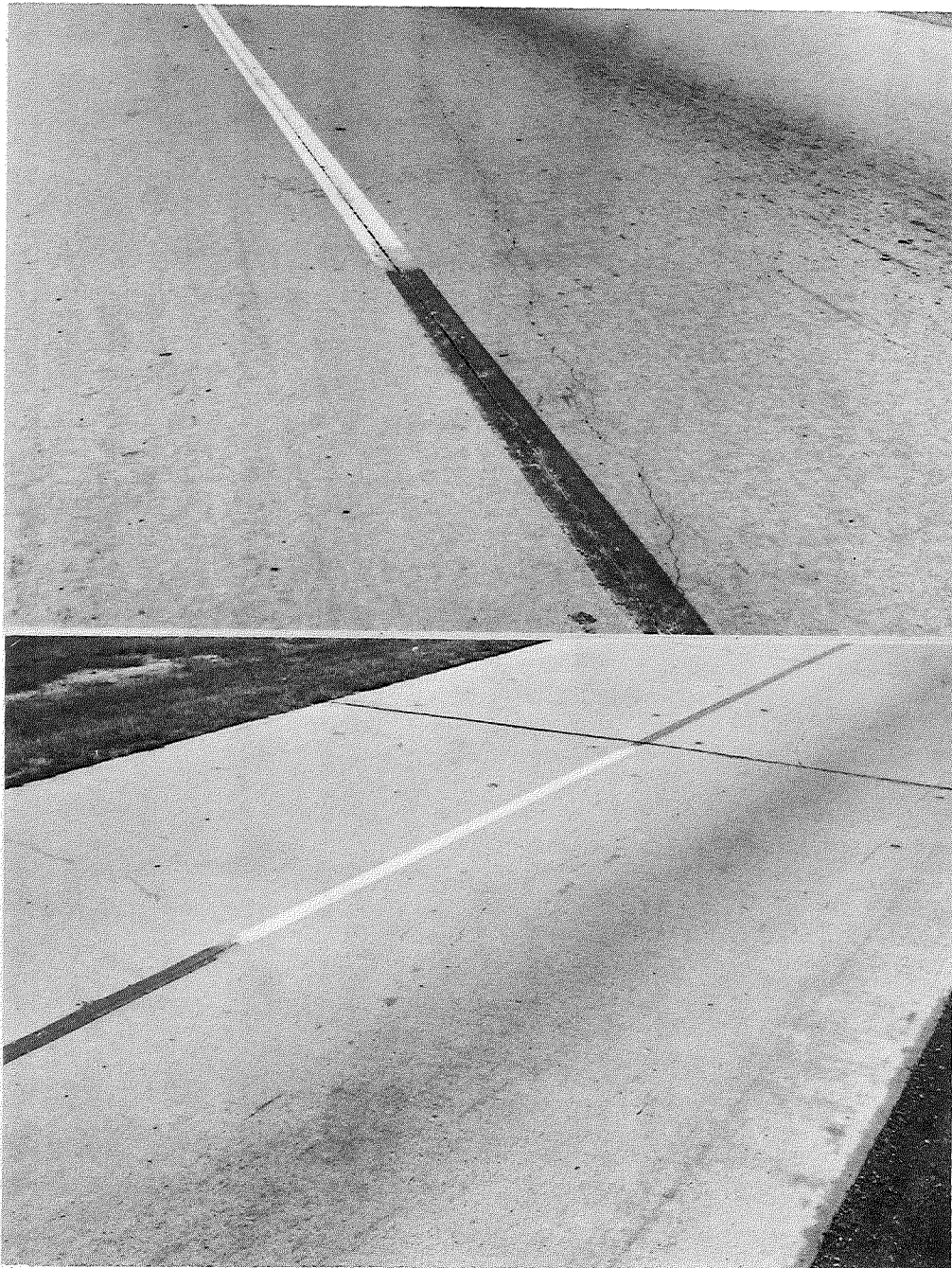
◀ Figure 1. Crack from centerline to pavement edge.
