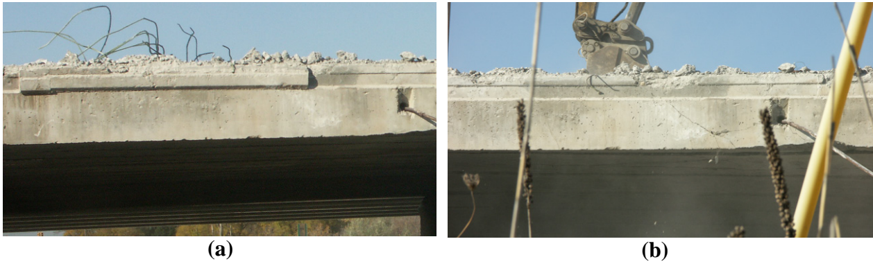
Figure 10-10. a) A portion of shear key grout remain intact with the beam and (b) beam surface after shear key grout cleanly fall off
