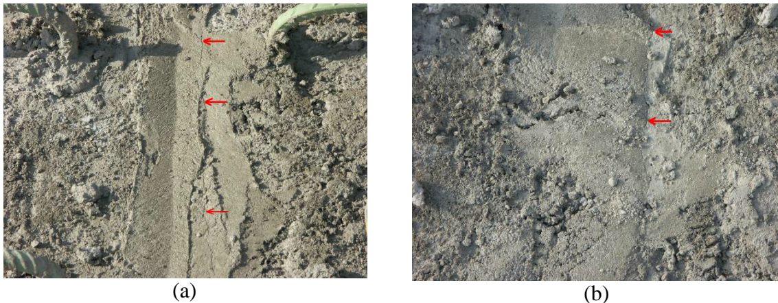
Figure 9-3. Shear-key interface cracking observed on May 14 th (a) before and (b) after posttension
