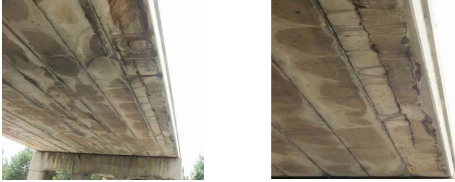
Photo 3-2. West fascia beam with full-length crack
