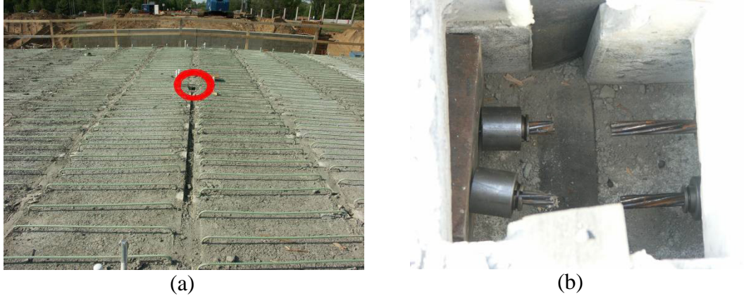
Figure 9-2. (a) Shear-key between beams 11 and 12 and (b) discontinued top posttension strands
