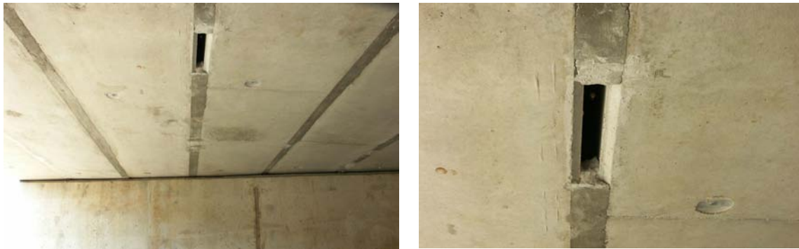
Figure 10-11. Shear key grout loss
