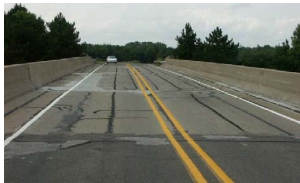
Photo 3-3. Wearing surface with multiple longitudinal cracks
