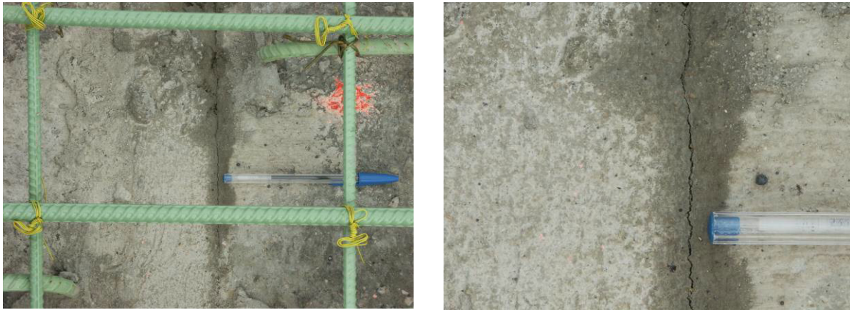
Figure 9-4. Shear-key interface cracks observed on June 4 th
