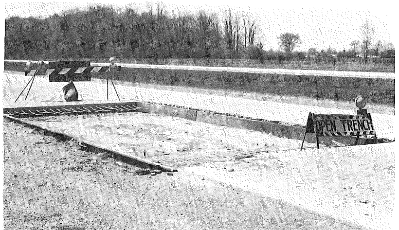
Figure 8. Condition of typical patch locations after removal of failed pavement, in bar mat section (top) and a welded wire mesh section (bottom).
