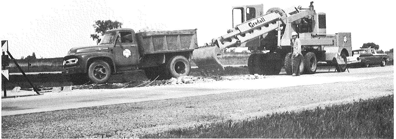
Figure 6. Removing concrete from a failed area, where both concrete and steel are to be replaced.
