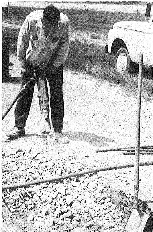
Figure 7. Breaking concrete with air hammer at the end of a patch, where 3 ft of original steel is to remain.
