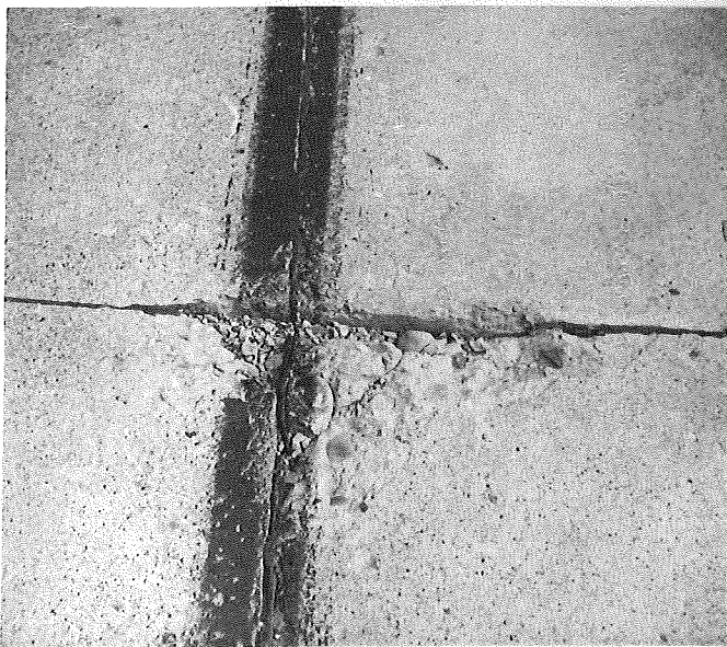
TYPICAL SPALLING OCCURRING ON SECTIONS WITH DOWELS. SERIES 1F, STATION 839+60.
