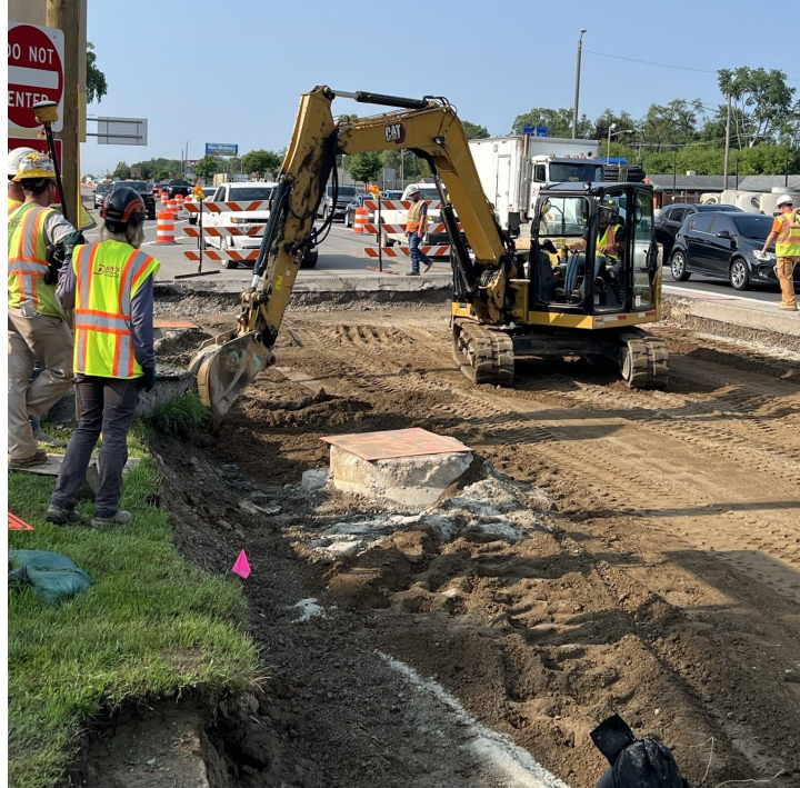
Figure 6.14. Mixing of Cement and Soil Using an Excavator in Tight Areas (Where a Rotary Pulverizer Cannot Reach) on US-24.
