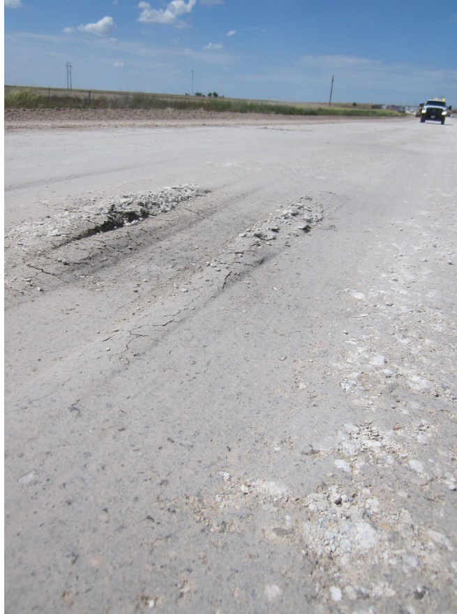
Figure 21. Location of Inadequate Stability Determined by Proof Rolling
