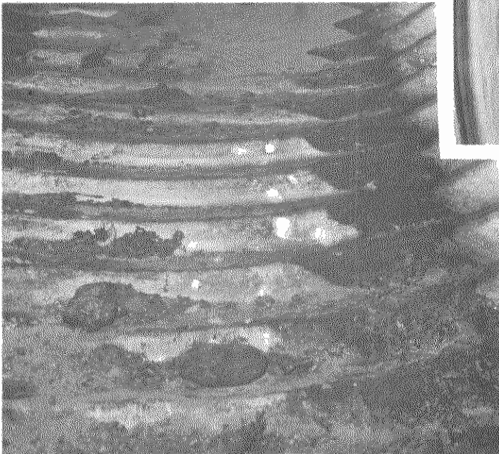
Figure 4. Aluminum culvert, Sta. 181+10. White spots near center are pitted areas that were beneath tightly adhering soil nodules. Pits apparently penetrated to the core alloy.
