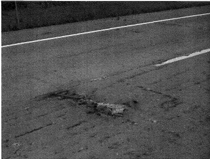
Figure 4. Corrosion of embedded steel.
