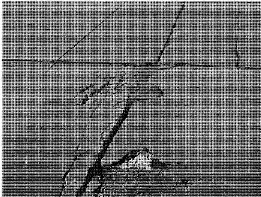
Figure 2. Cracking, staining, and spalling at joint.
