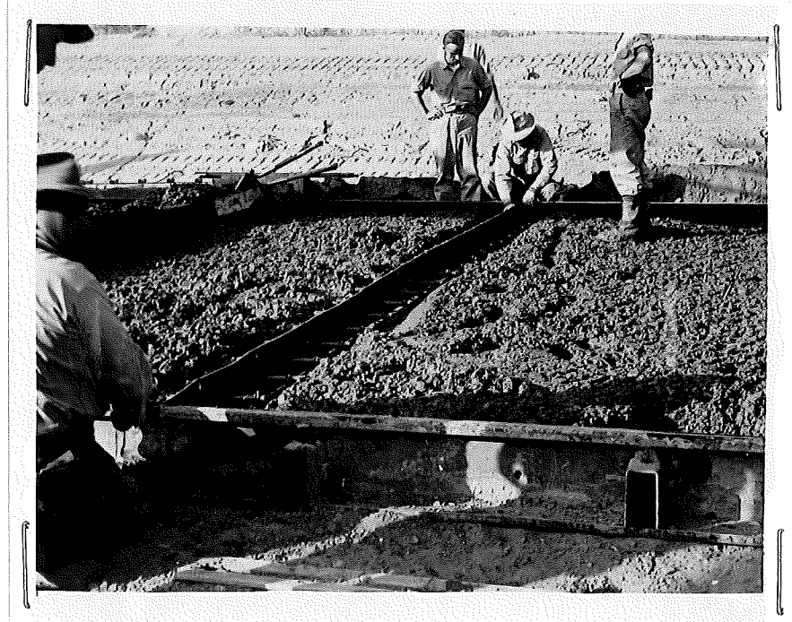
Figure 13. Early stage during installation of precompressed and treated redwood contraction joint assembly at Station 779 + 68. Joint assembly being trued to form and crown.
