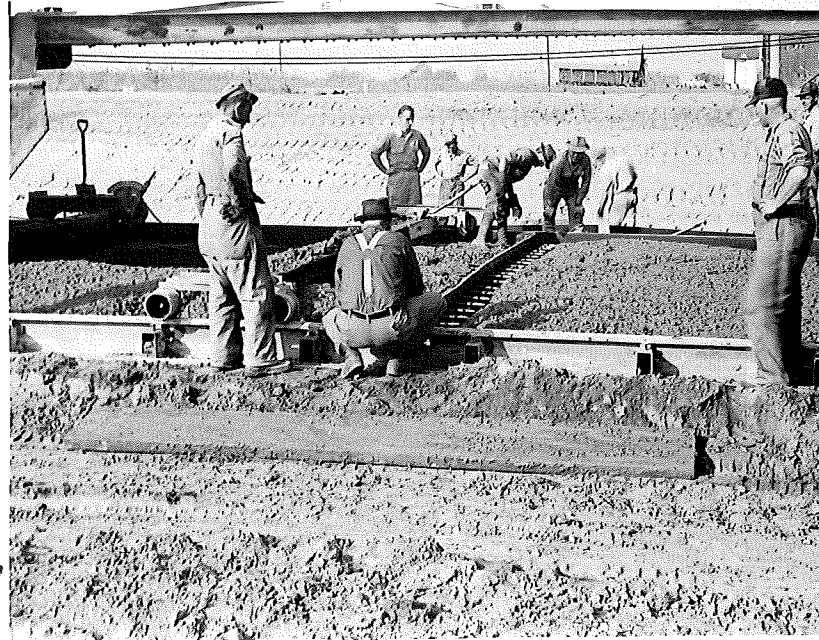
Figure 11. Stage during installation of experimental precompressed and treated redwood expansion joint assembly at Station 780 + 68. Assembly is being trued to form.
