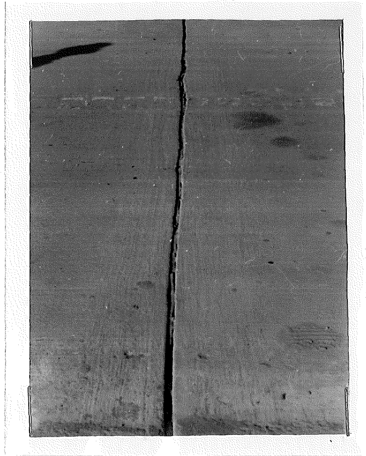
Figure 15. Shows condition of redwood contraction joint at Station 778 + 68 three weeks after installation.
