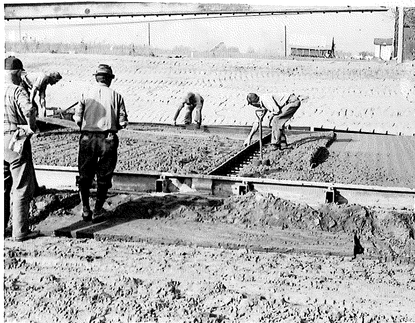
Figure 12. Stage during installation of experimental precompressed and treated redwood expansion joint assembly at Station 780 + 68. Steel reinforcing mesh being placed over first layer of concrete west of joint. Note care being taken to avoid displacement of joint assembly.
