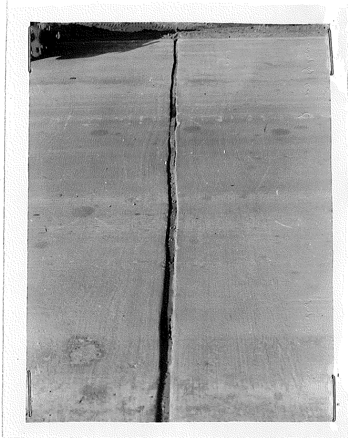
Figure 16. Shows condition of redwood expansion joint at Station 780 + 68 three weeks after installation.
