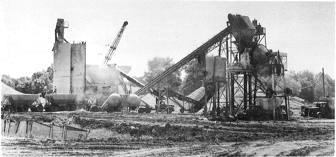
▲ Figure 1. General view of batch plant and mixer.
