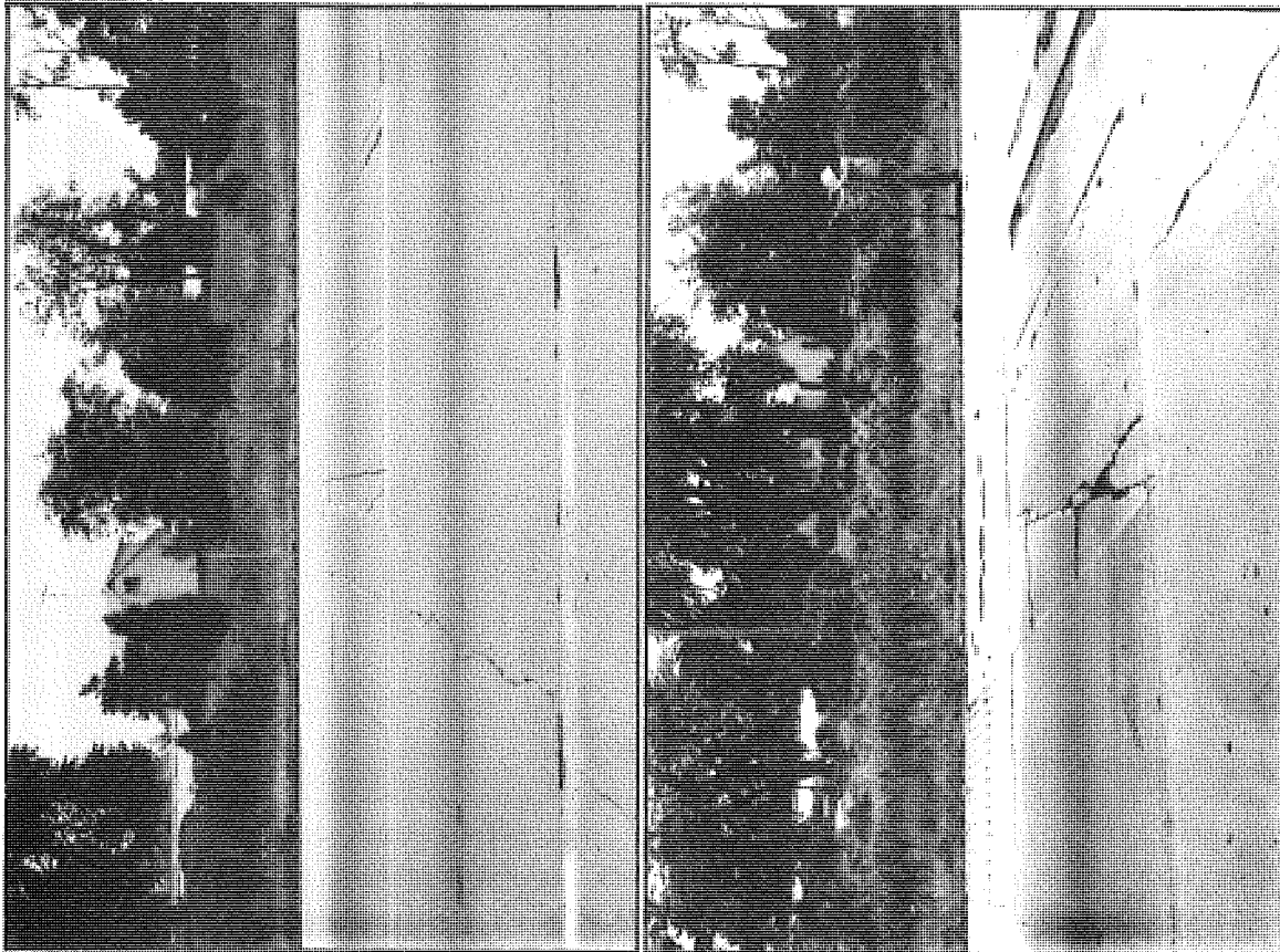
Figure 4. Typical distressed areas illustrating the maximum and minimum range of differential movement of the surface of the add-on lane compared to the adjacent shoulder.
