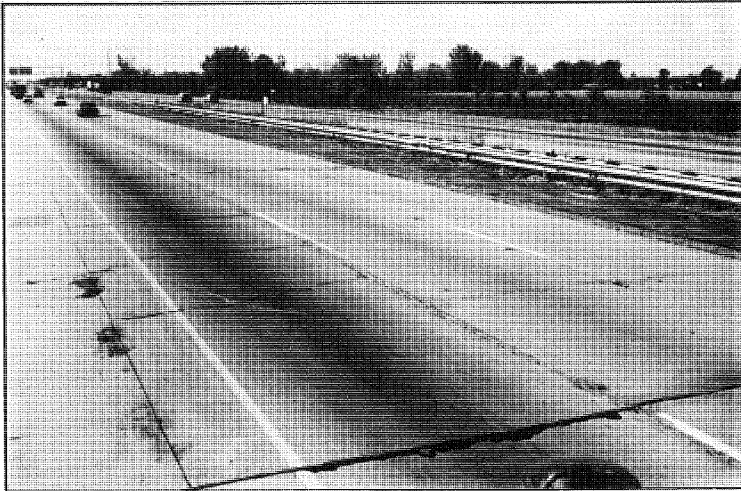
Figure 11. Moderate transverse cracking and faulting. Add-on lane is depressed compared to original pavement indicating there is no bond between them.
