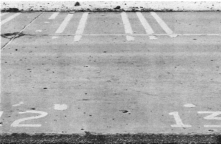
▲ January 21, 1959, after 447 days exposure, with passing lane striping exhibiting much better service than traffic lane striping.
