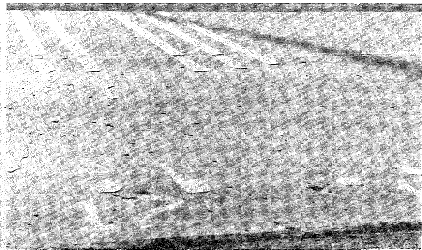
▲ February 25, 1958, after 150 days exposure, showing complete loss of striping in traffic lane.
