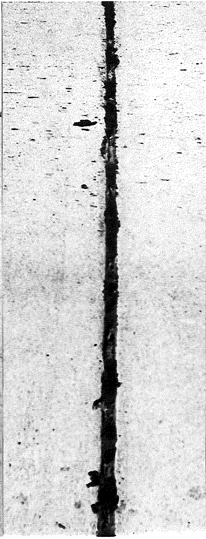
▲ FIGURE 3. JOINT SEAL IN FAIR CONDITION. NOTE ALTERNATE GOOD AND BAD AREAS. STONES IN JOINT. STATION 29 + 60 NORTHBOUND.
