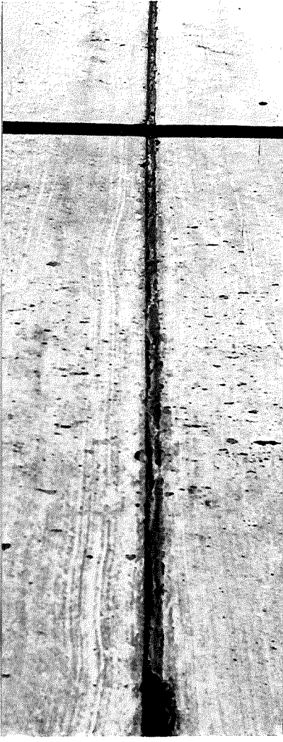
▲ FIGURE 4. JOINT SEAL IN GENERALLY POOR CONDITION ALONG ENTIRE LENGTH OF JOINT. STATION 53 + 25 NORTHBOUND.
