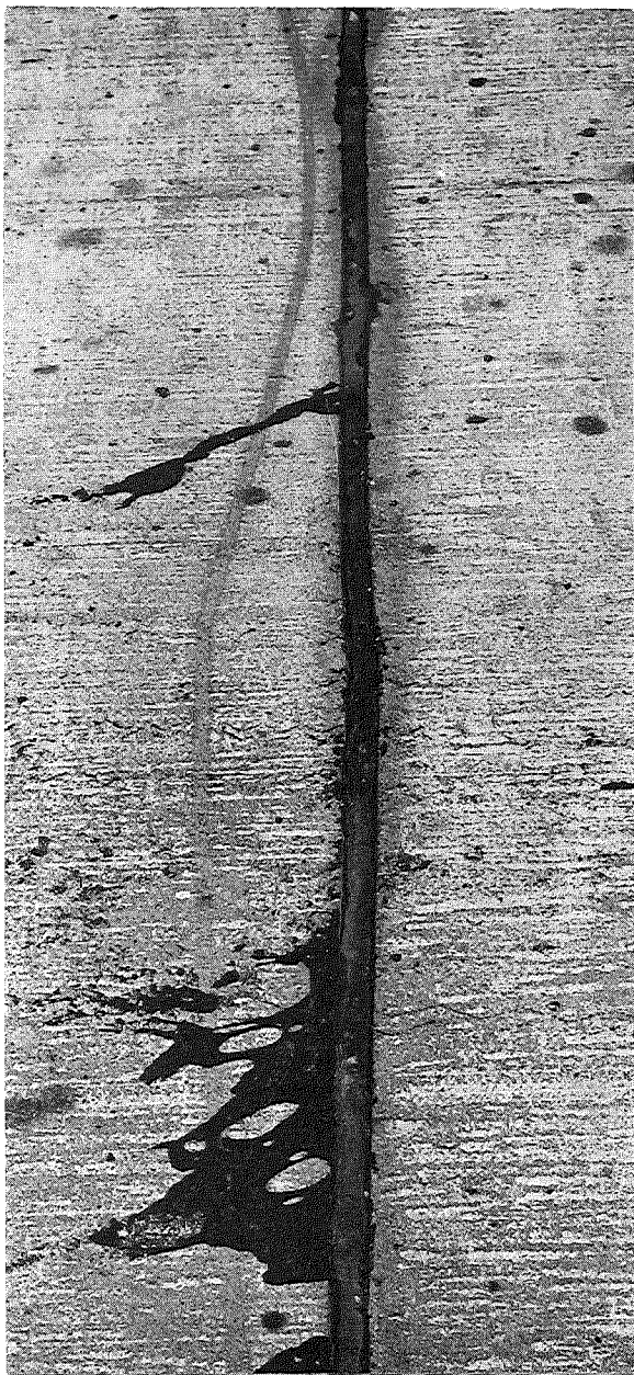
Figure 4. Typical severe adhesion failure with embedded dirt (Project BI 50112A, C1, Sta. 798+02 NB).
