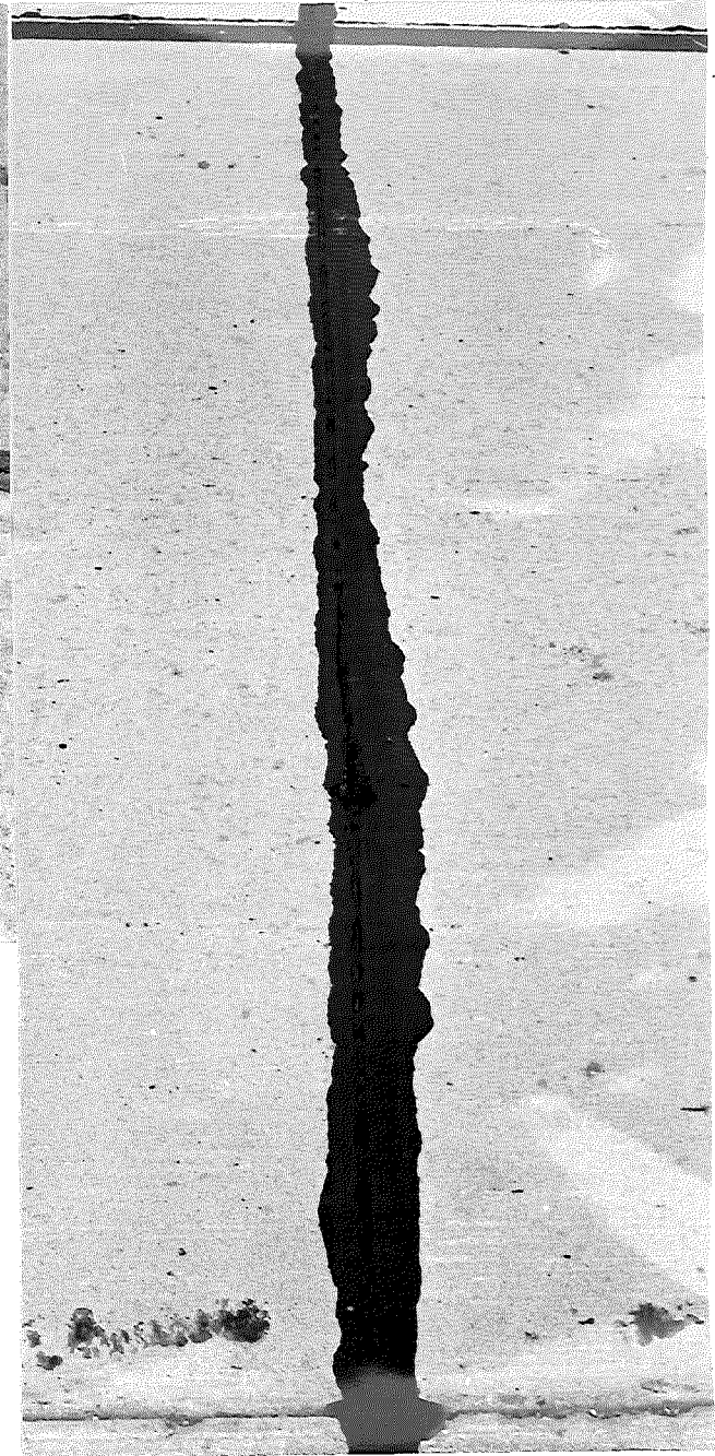
Figure 1. Joint sealant appearance in November 1963 (left), and June 1964 (right) showing exuded warm weather condition and healing of cohesion failure (Sta. 343+80 SB). Same joint shown in Fig. 2 of Research Report R-456.
