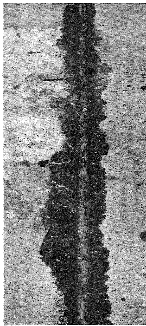
Figure 6. Overfilled joint with typical cohesion - adhesion failure (Project BI 77111B, C3, Sta. 1203+50 NB).
