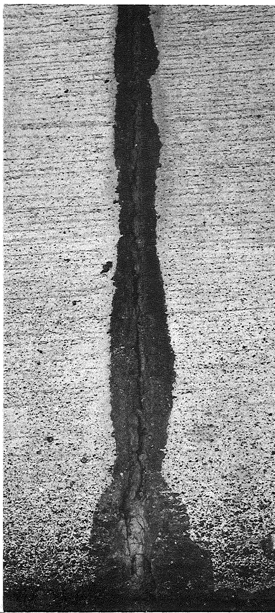
Figure 5. Cohesion failure typical of this area (Project BI 77111A, C2, Sta. 908+02 NB).
