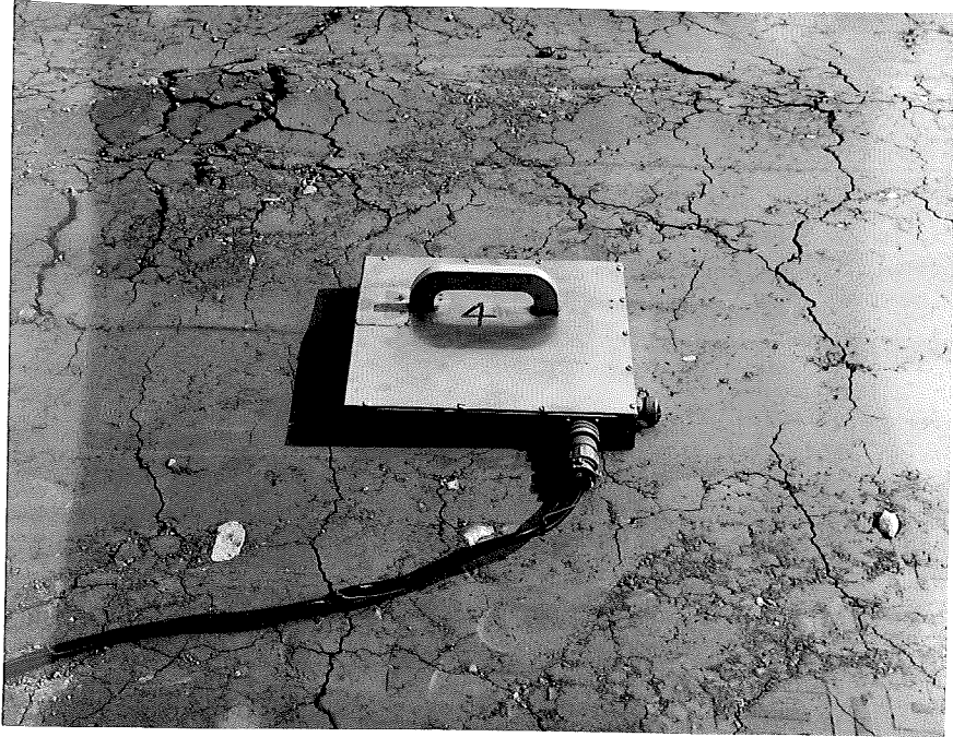
Figure 9. Cracking of compacted surface in moist areas (nuclear density gage shown in place).
