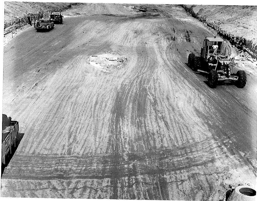
Figure 8. Uneven moisture distribution after compaction.
