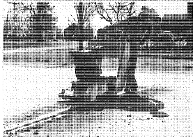
Figure 3. Sargent used Windsor router (top) for routing and scarifying, and then cleaned further with rotating wire brush (bottom).
