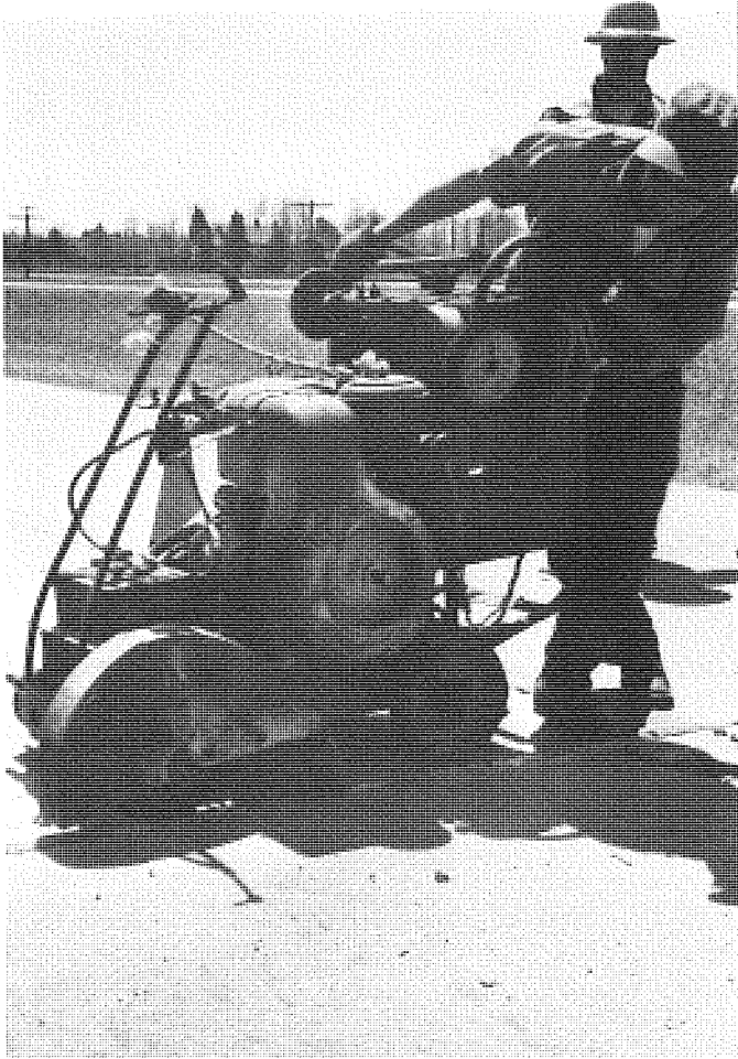
Figure 2. Barton's only mechanical operation in cleaning joint groove and scarifying joint faces was concrete saw containing spaced vertical carborundum blades.
