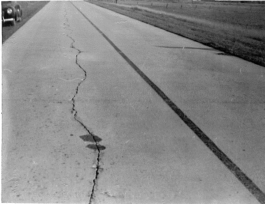
Figure 3. Typical longitudinal cracking, Station 330+00.
