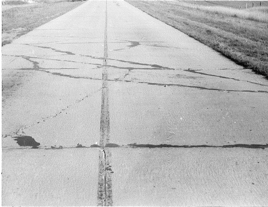
Figure 8. View of cracking over culvert at Station 258+50.
