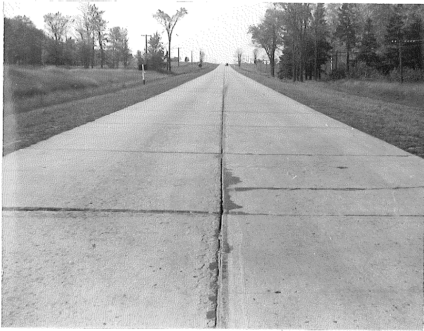
Figure 4. Opening of center joint where tie bars were not used, Station 396+50 to US-2.
