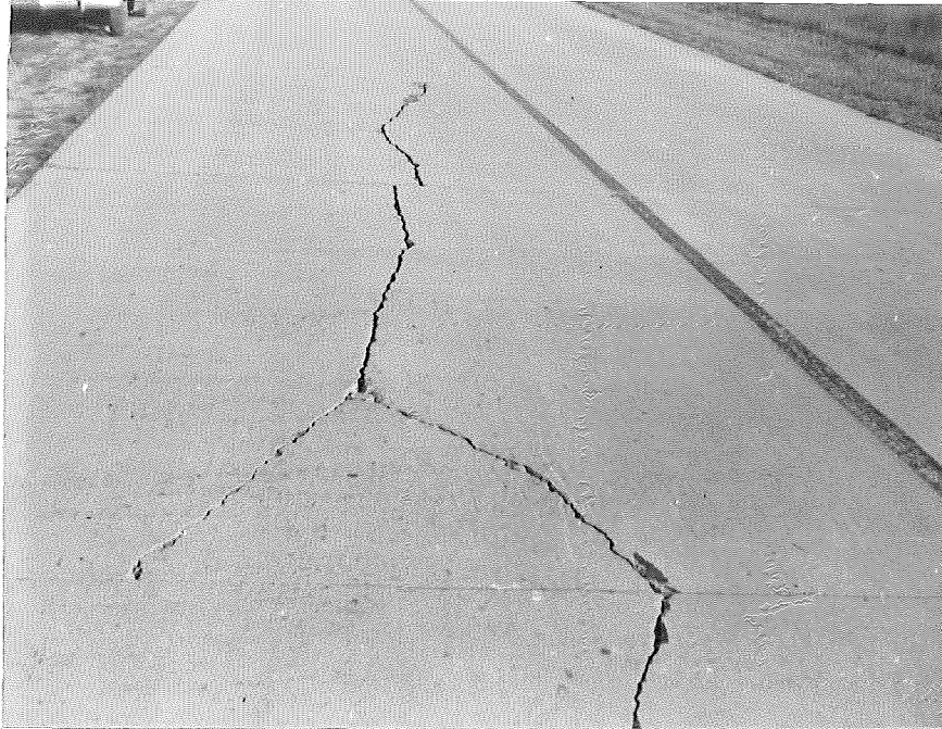
Figure 2. Typical longitudinal cracking, Station 325+50. Note width of cracks.
