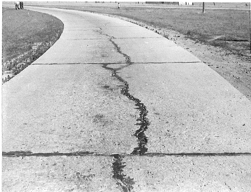
Figure 9. Typical cracking of 14 foot width pavement forming north leg of Wye at intersection with US-2.
