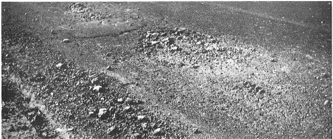
Figure 4. Behavior of asphalt leveling course, showing severe alligator cracking (top) and localized distress (center and bottom).
