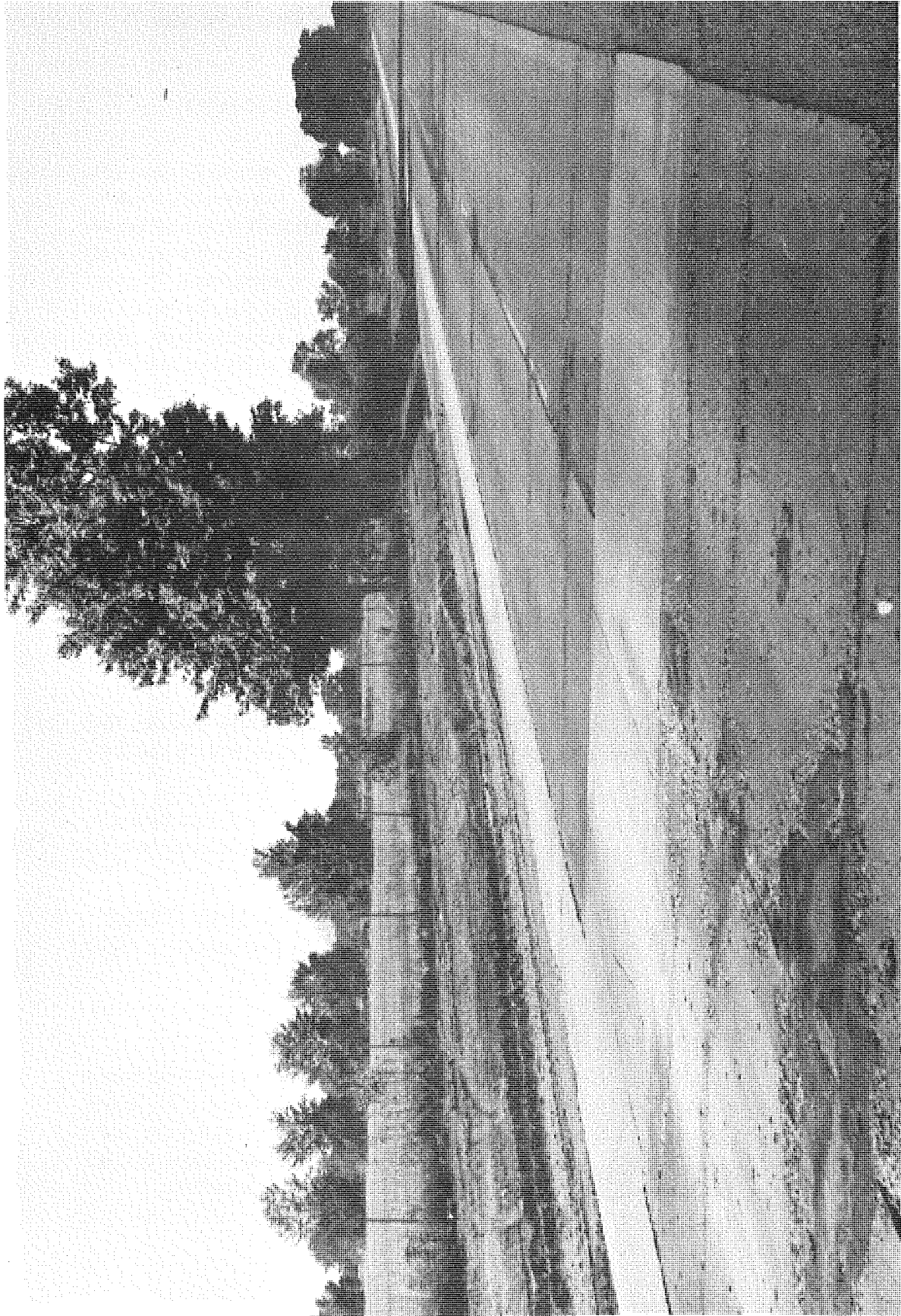
Figure 1. Original rigid pavement. Note transverse patch replacing blow-up.
