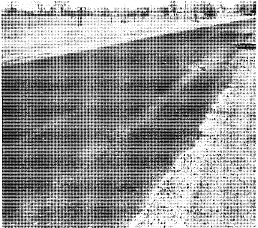
Figure 3. Behavior as asphalt leveling course, showing map cracking and disintegration (upper right), longitudinal cracking and disintegration (lower left), and moisture spotting (lower right).
