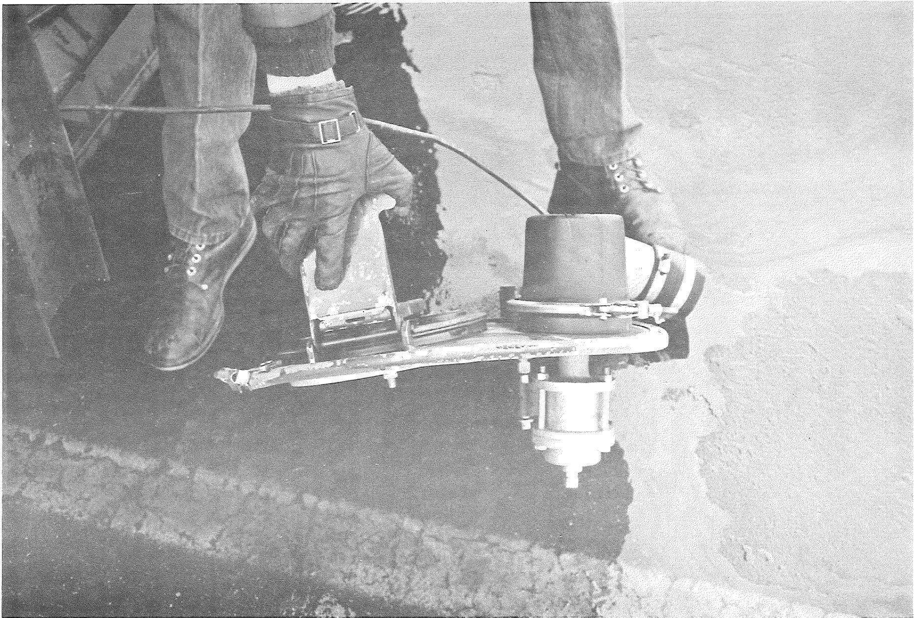
Figure 5.24. Failed manhole cover showing bowed profile.
