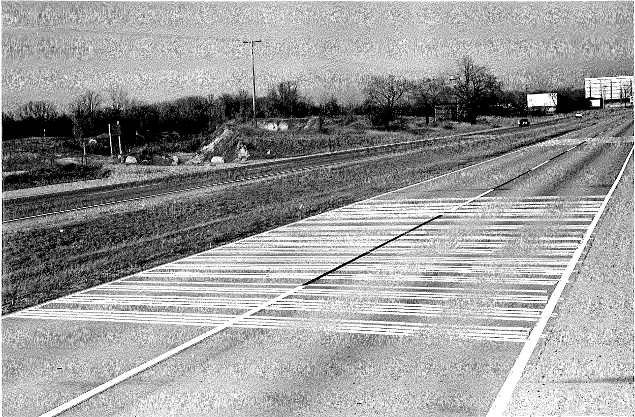
Figure 3. General view of strip appearance at end of ratings. These were in somewhat poorer condition than the stripes on the bituminous pavement. The 1971 fast-dry test stripes (concrete) can be seen in the background.
