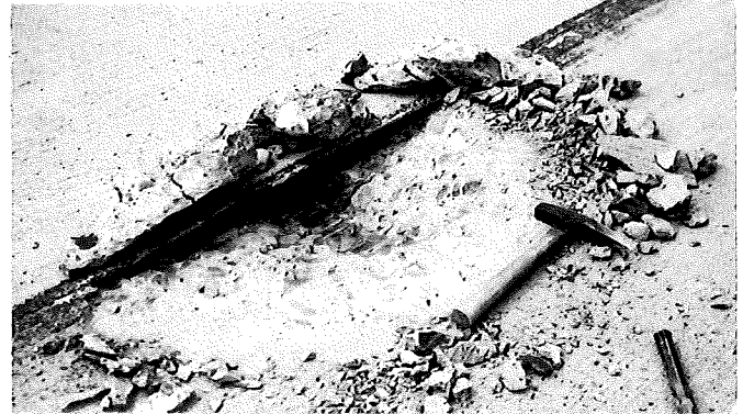
▲ FIGURE 11 - SPALL AT CENTER JOINT, STA. 225+92 -F7-20, C6. NOTE TWO REINFORCEMENT BARS AT BOTTOM OF SPALL.
