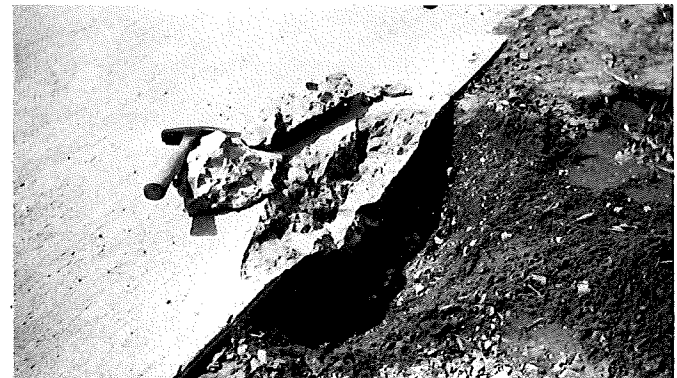
▲ FIGURE 13 - SPALL AT PAVEMENT EDGE, STA. 228 + 38 LT. F7-20, C6.
