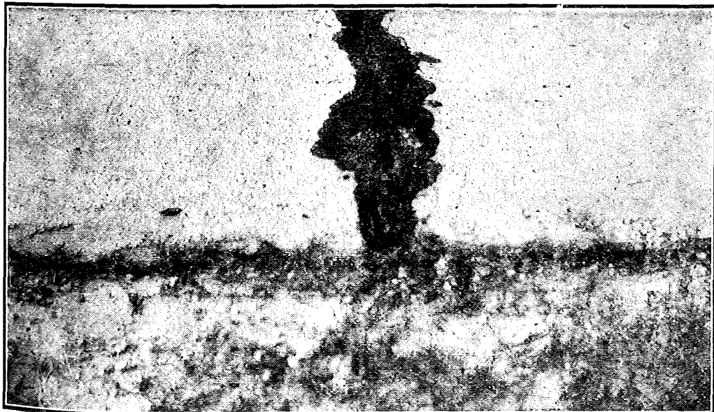
FIG. 3.—ASPHALT BURNED OUT OF JOINT AT POINT OF ARC.
