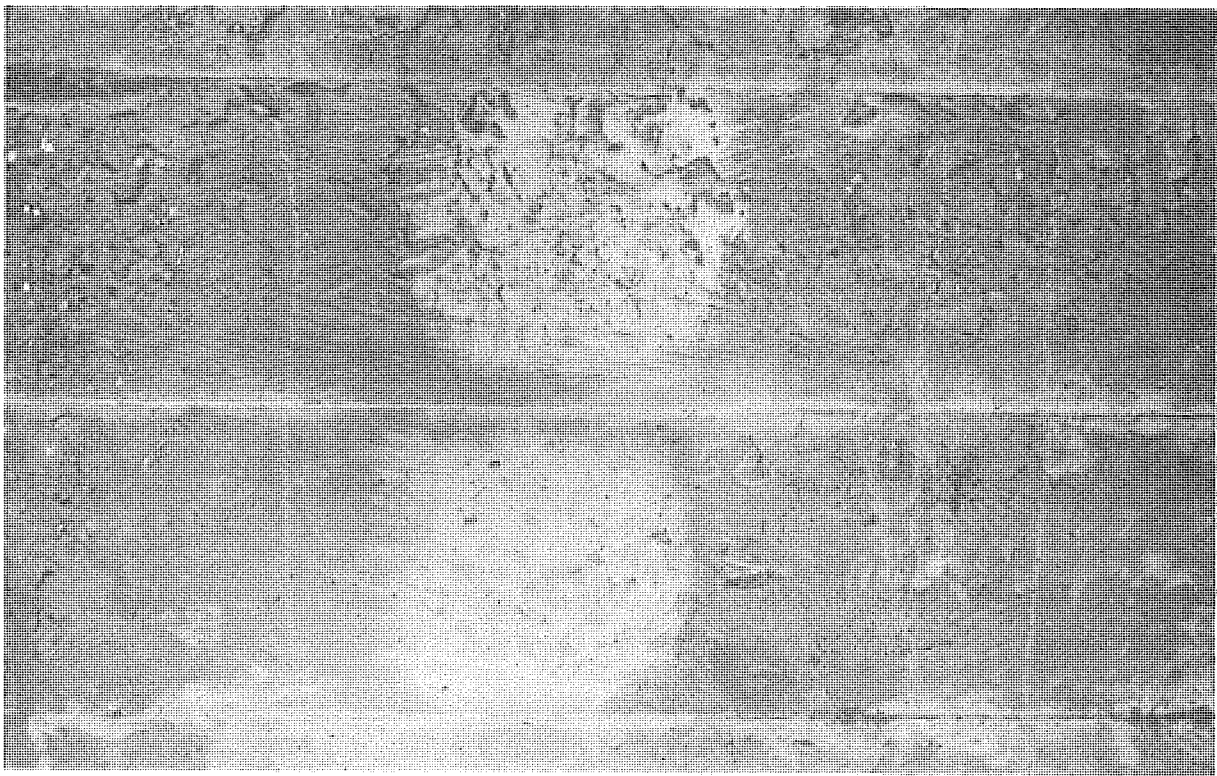
Figure 4. West arch-rib hammer reading positions 55 and 56 before and after surface preparation. Note variability of surface texture between the two positions.
