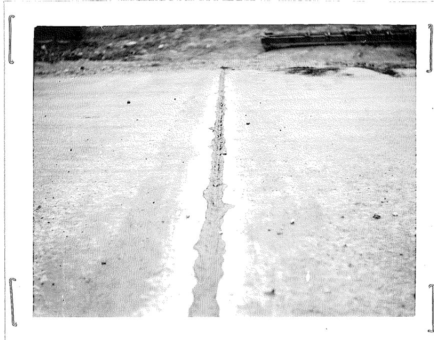
Illustration No. 6 Poor joint at Station 432+00 near junction of M-46 and M-19
