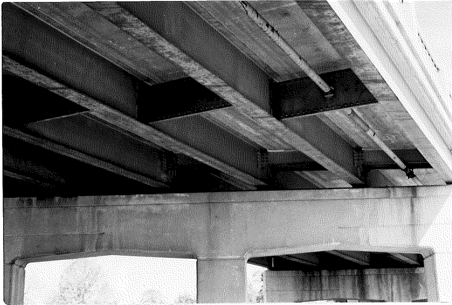
Figure 1. Condition before repainting of original paint system on test bridge. Paint system was 11-yr old.
