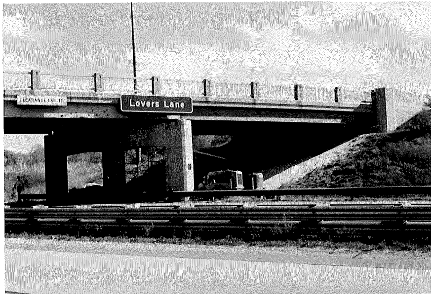
Figure 2. Beginning of repainting operation on south end-span of test structure. The brown paint (right) is newly applied by the electrostatic spray equipment.
