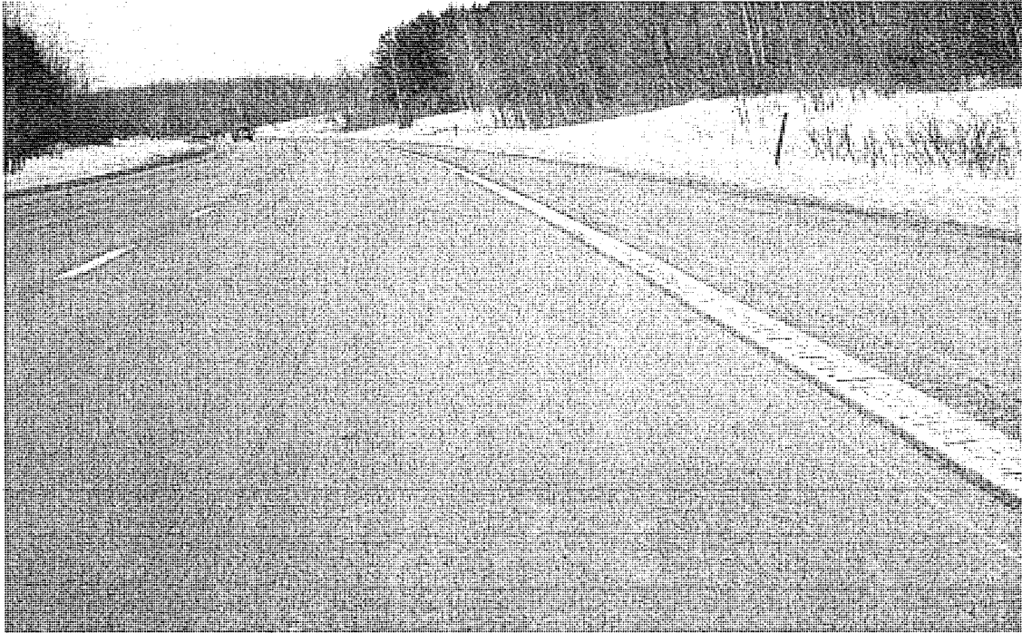
Figure 37. Performance of white 6-in rumbled edge line on Northbound US-131 after winter maintenance, February 15, 2004.
