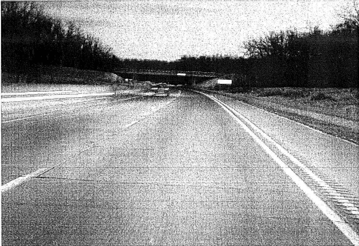
Figure 41. Performance of white 4-in rumbled and solid edge lines on Southbound US-131 after winter maintenance, February 15, 2004.
