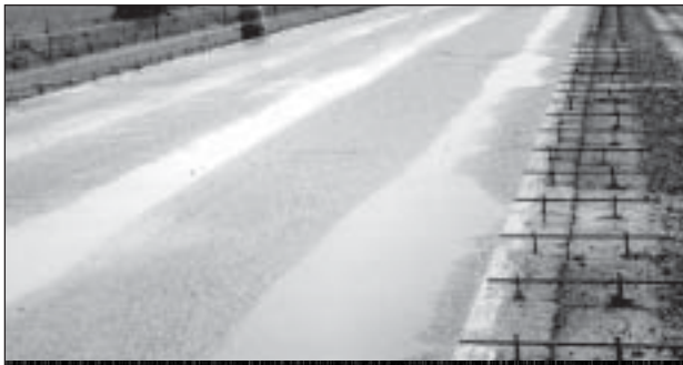
Figure 2. Rutting in existing pavement (note lane tie placement on the right shoulder)
