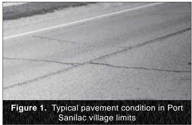
Figure 1. Typical pavement condition in Port Sanilac village limits
