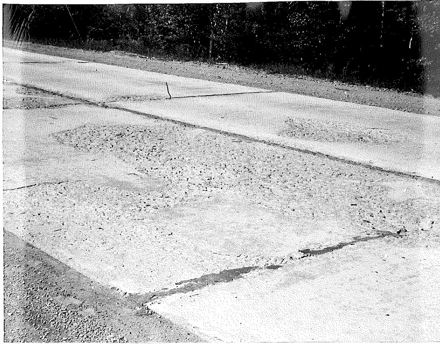
Fig. 8 Typical scaling and pitting at Station 34+00.
