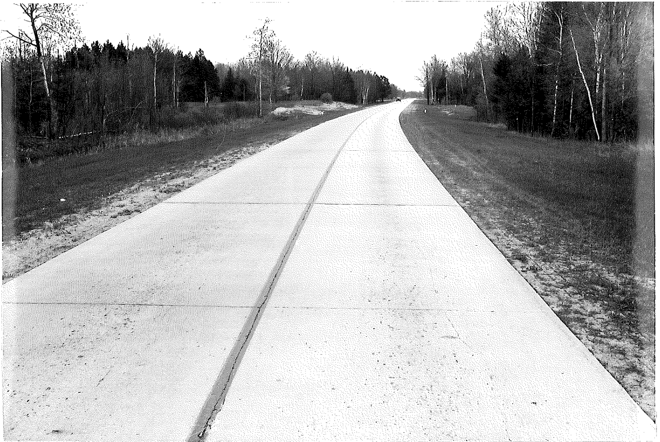
Figure 2. General view of durability project section containing Pozzolite. Taken at middle of section looking south. Note absence of scaling.
