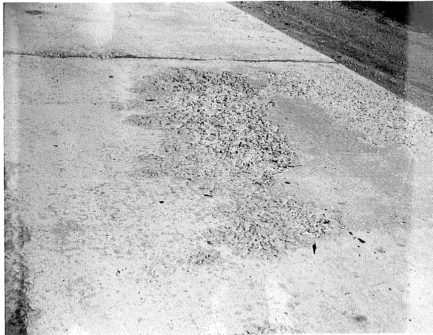
Fig. 7 Character of scaling and deep pitting 33+00.
