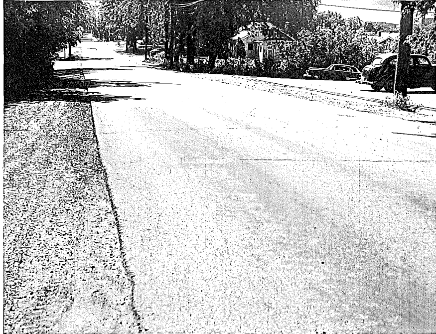
A. General view showing close texture. No pitting.
