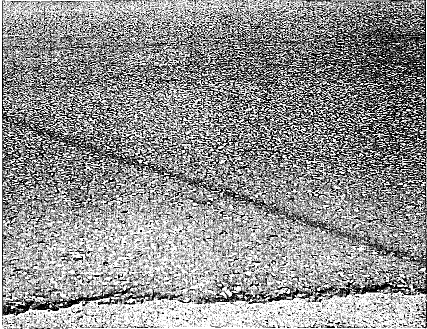
A. Condition of surface showing slight pitting.
