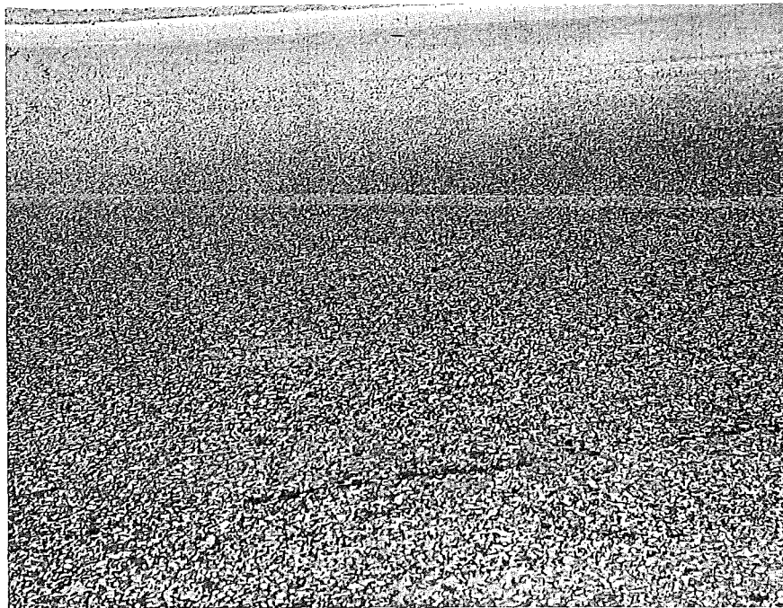
A. Condition of surface. Slight pitting.
