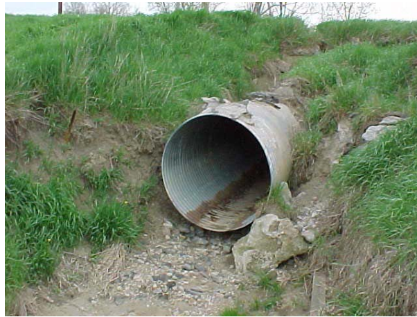
Riprap condition rating of 3 or less (Material has failed, significant loss of embankment).
