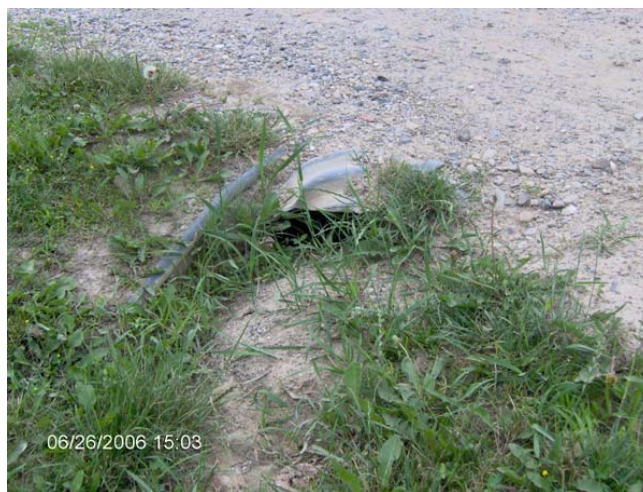
Sediment blocking more than 50% of culvert depth –condition rating of 3 or less
