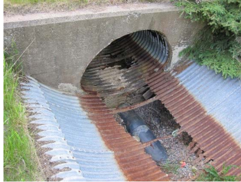
Condition rating 2 or less
