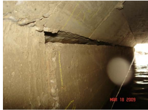
Slab culvert with failed wall Condition rating 3 or less
