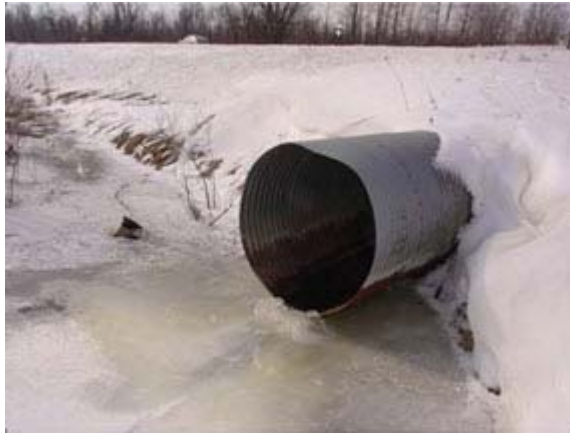
Perched culvert (culvert invert above channel invert) – condition rating of 3 or less
