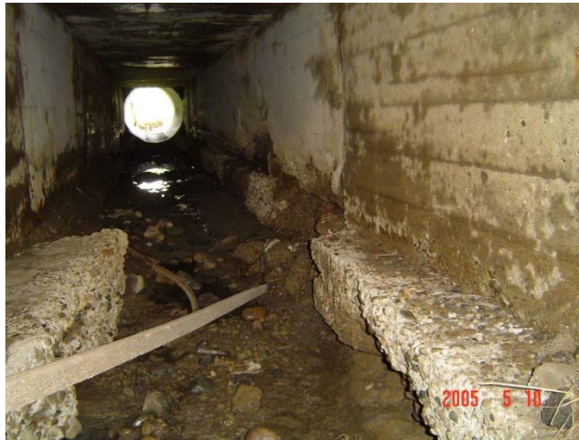
Example of culvert that has been extended multiple times (note different material and shape of current outlet when compared to the existing culvert).
