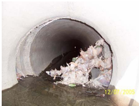
Joint separation in culvert- condition rating of 3
