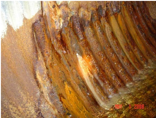
Significant rust with section loss Condition rating 3 or less
