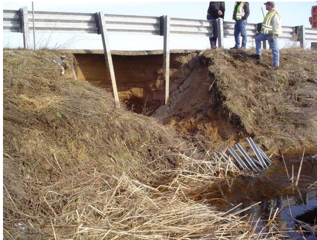
Embankment has failed is affecting traffic - condition rating of 2 or less.
