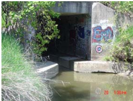
Footings significantly exposed – condition rating 3.
