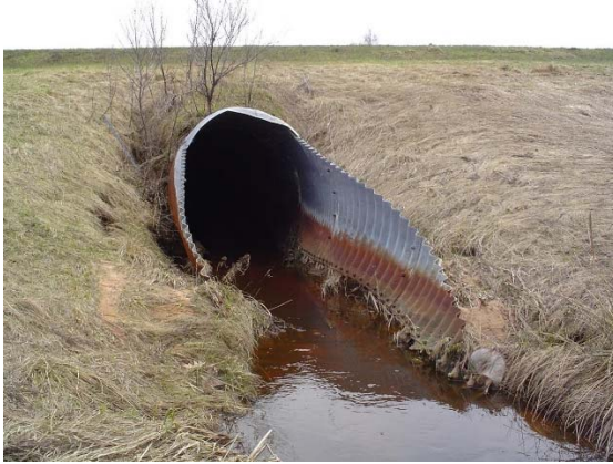
Condition rating 6 or less
