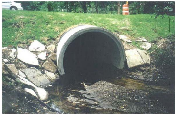
Riprap condition rating of 5 or less (poor material, non-interlocking, only 1 layer remaining).
