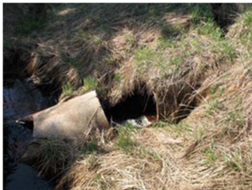
Detached end section- condition rating of 3.
