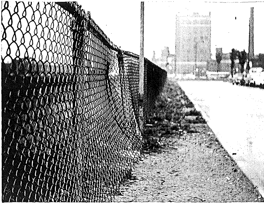
Figure 1. Galvanized steel fence damaged by vehicle (east service drive between Madison and Clinton Avenues. Walter P. Chrysler Expressway, Detroit).
