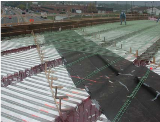
Figure 6.31. Installation of link slab formwork and continuous reinforcement throughout link slab and adjacent concrete
