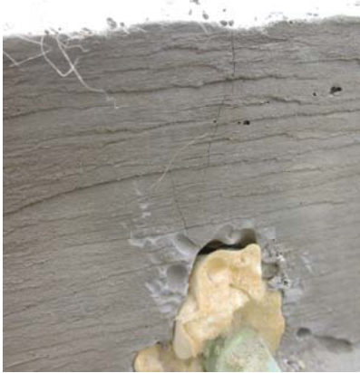
Figure 6.20. Cracking in ECC link slab cross section at reinforcing steel with width 0.007" at surface. (8 Days)
