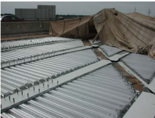
Figure 6.3. Painting of girders after installation of new shear connectors. Notice lack of shear connectors within link slab debond zone.
