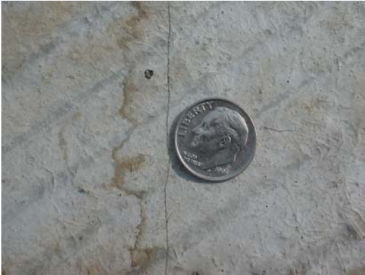
Figure 6.16. Cracking within ECC link slab with crack width approximately 0.007". (3 Days)
