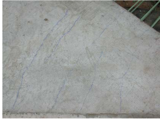
Figure 6.19. Cracking in ECC link slab (highlighted with blue chalk) corner with crack width 0.005. (8 Days)
