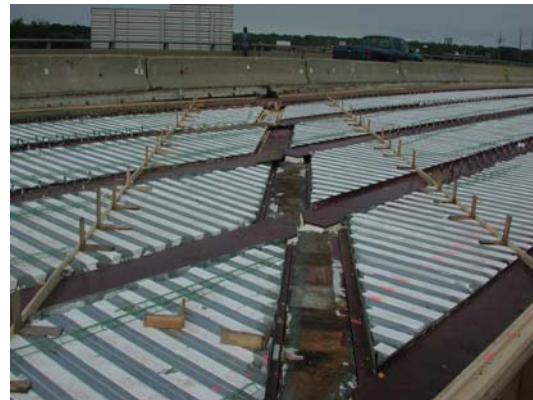
Figure 6.4. Preparing formwork for placing of conventional deck adjacent to each side of ECC link slab.
