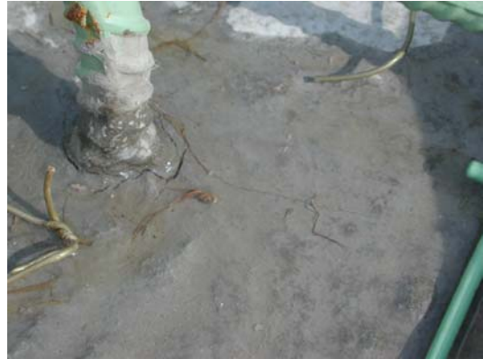
Figure 6.17. Cracking in ECC link slab around sidewalk reinforcing steel with crack width approximately 0.014". (3 Days)
