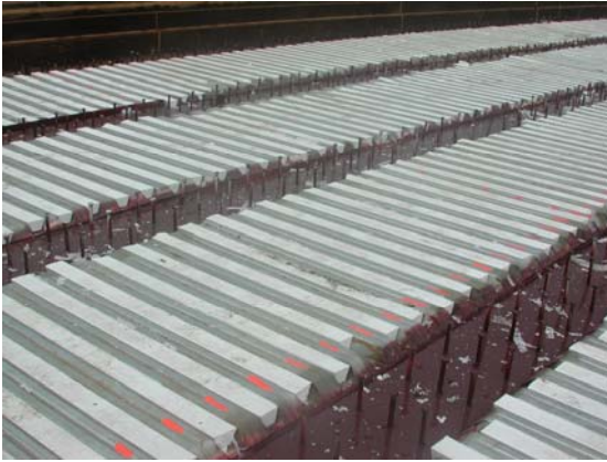
Figure 6.29. Completion of stay-in-place formwork, painting of girders, and installation of new shear connectors.
