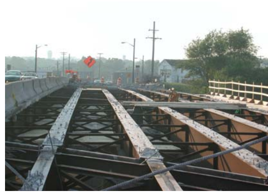
Figure 6.2. Exposed steel girders with shear studs removed.
