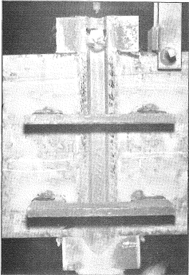
Figure 9. Completed electroslag weld with retaining shoes removed, strong-backs, sump and tabs still in place (Bridge Shop C).
