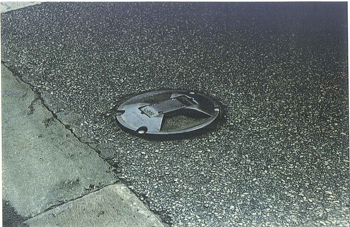
Figure 10: “Runway” lighting to help illuminate the turning path. Note the buildup of debris.
